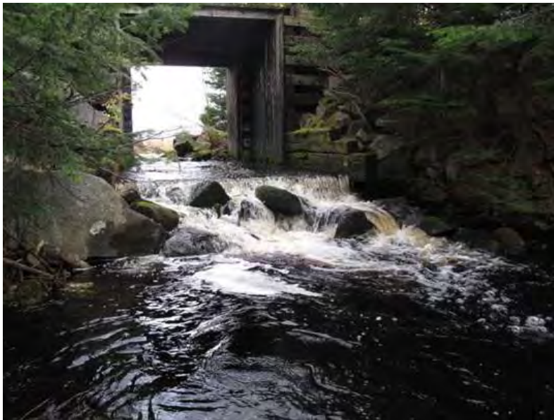
Photo 1 Barrier to Fish Passage Structure at Entrance to Nashwaak Lake.
