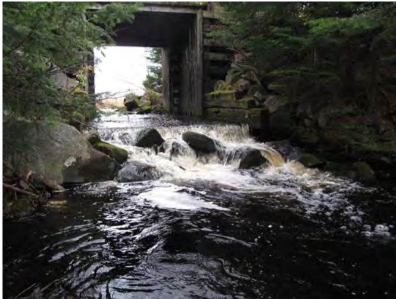
Photo 7.4.1 Barrier to Fish Passage Structure at Entrance to Nashwaak Lake.
